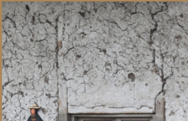
figura 139. Fisura vertical* Gualaceo - Azuay
