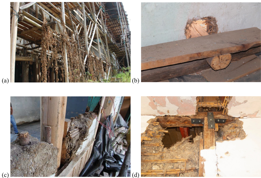
Fig. 5. (a) Scaffolding system affecting various parts of the structure. (b) Pathology structural intervention in walls of wattle and bahareque walls to support scaffolding systems. (c) Cutting and breaking of wooden parts. (d) Reinforcement of metal profiles. Source: Own (2020)
