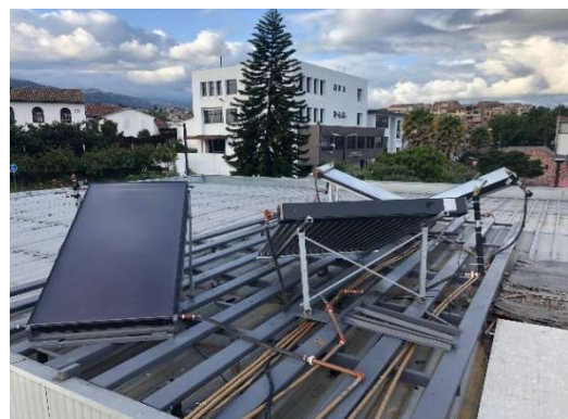
Fig. 1. Solar collectors installed at different orientations and inclinations.
