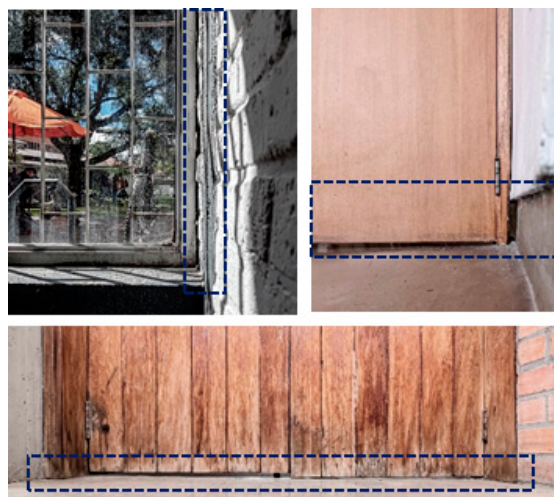
Figure 7. Envelope encounters with classroom windows and doors.
