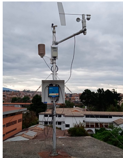
Figure 2. Delta T GP2 weather station on the roofs of the buildings at the Faculty of Architecture.
