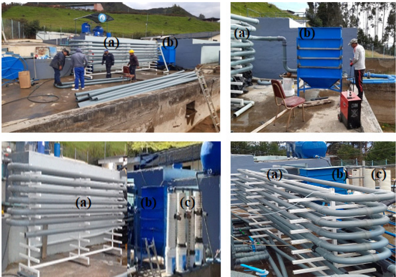
Figure 13. Implementation of the Pilot Treatment System. The upper left figure shows the HTF implementation; in the upper right, the implementation of the settler is presented. The complete experimental system is presented in the lower left and right figures, as follows: (a) HTF, (b) high-rate settler, and (c) rapid sand filters.
