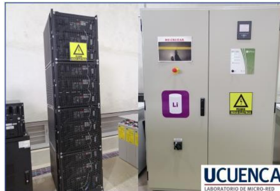
Figure A1. Lithium-ion BESS from the micro-grid laboratory: cell bank (left), power electronics converter cabinet (right).
