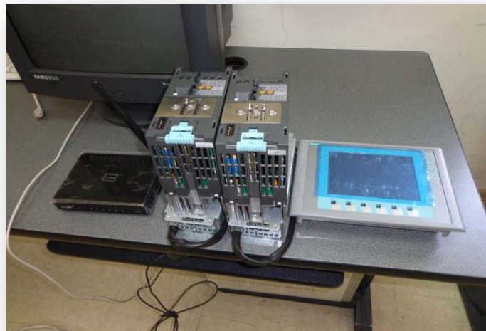
FIG.125 HMI KTP600, DRIVE G120, Router TP-Link 600
