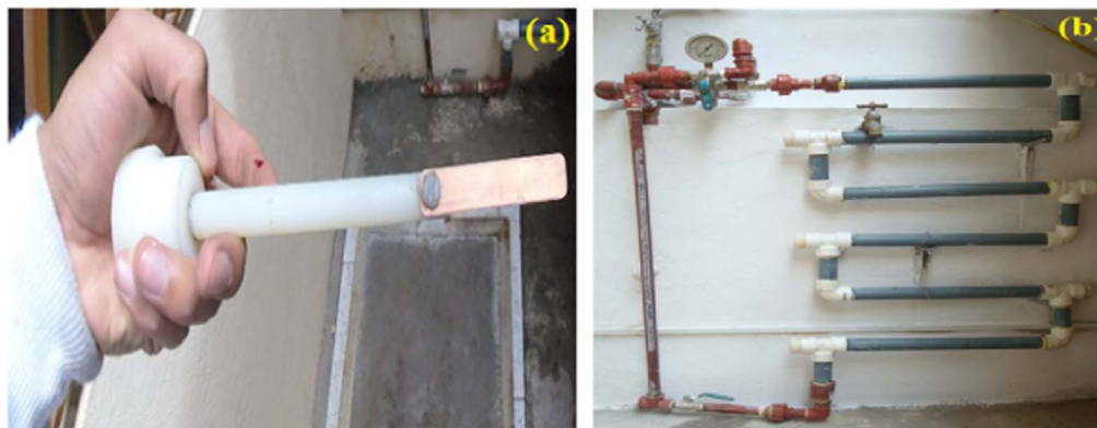
Fig. 8. Installation of copper coupons in a domicile (a) Coupon holder (b) Corrosion test rack.
