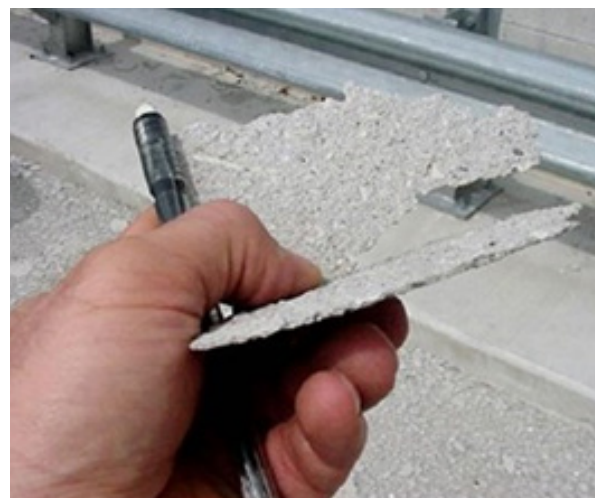
Figura 39. Delaminaciones (George W. Seegebrecht, ConcreteNetwork.com)
