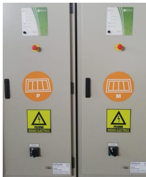
Figura 3.5 Inversor GPTech PV15. [Elaboración propia, 2022]
