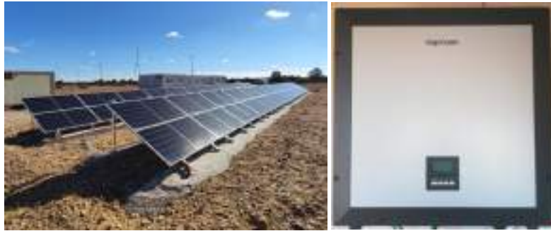
Fig. 2. Photovoltaic system (photovoltaic modules and DC/AC inverter).
