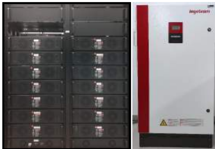
Fig. 4. LFP battery rack and inverter.
