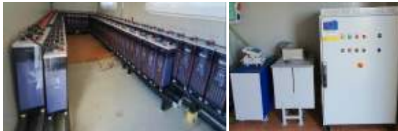
Fig. 3. Lead-acid batteries and DC/AC inverter.
