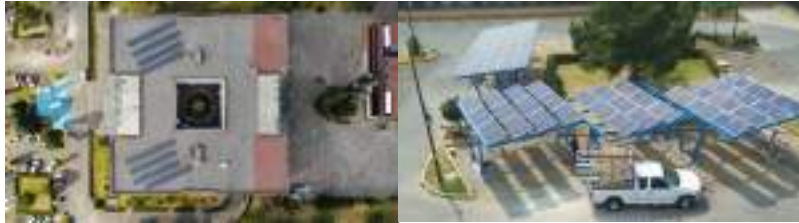
Fig. 1. SPV electricity generation plant installed at CIC-IPN.
