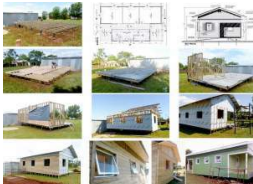
Fig. 2. Floor plan, elevation and photographs of the construction phases of INVICO's viviendas sociales at the Virasoro locality. [© INVICO (drawings) and Erick Kennedy (photographs)]
