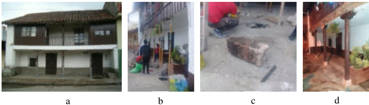
Figure 5: Juárez House (O409); main facade before the intervention; b) shoring of the portal during the replacement of the bases; c) original unburied bases; d) columns after the intervention Source: a) Photographical archive of the Municipal Foundation “El Barranco”; b,c,d) Photographical archive of the World City Heritage Project, 2018
