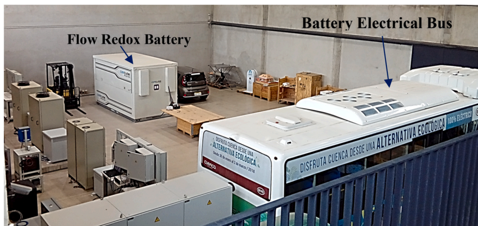
Fig. 14. Test bench, with BEB and Flow Redox Battery.
