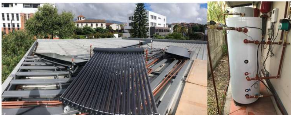
Figure 3. Photographs of the installation of one of the STCs and a storage tank taken from the south.
