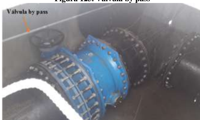
Figura 123. Válvula by pass
