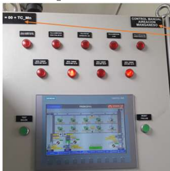
Figura 9. Tablero de control = 00 + TC_Mn – CONTROL MANUAL AIREACIÓN MANGANESO
