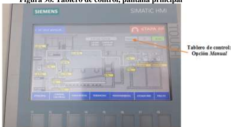
Figura 98. Tablero de control, pantalla principal
