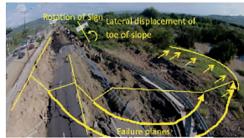
Figure 6: Failure of the Mejia Bridge (EERI, 2016)
