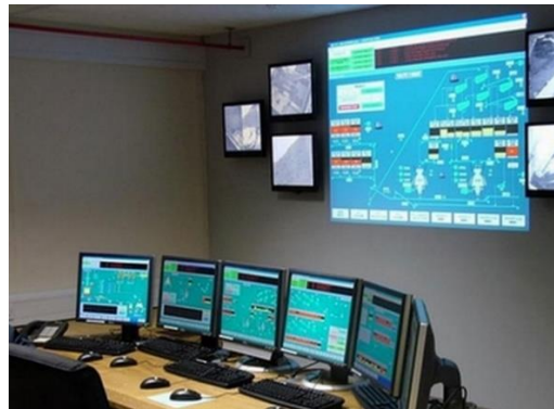
Figura 2.6.10 Centro de control. (Fuente: https://www.cyberinject.com/what-is-scada/ ).
